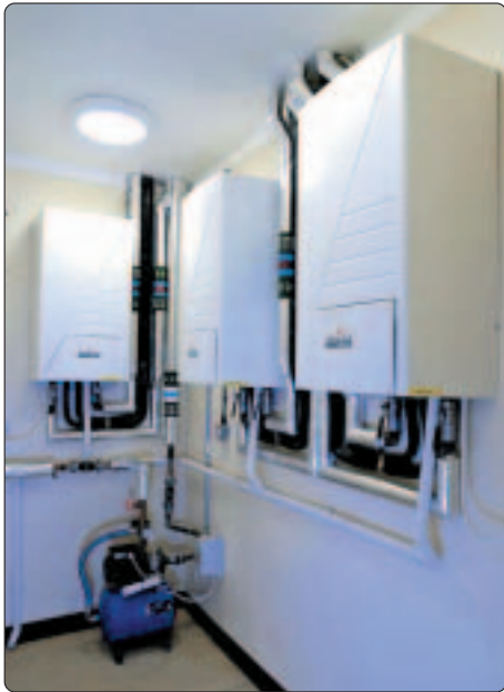
Three Altherma air to water split heat pump systems, supplied by Daikin Airconditioning UK Ltd, specified by Helix
